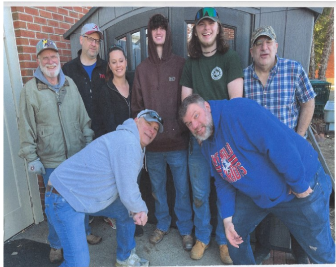
Nashua Elks Lodge 720 /NH-ENVSC members furnished and installed a new shed at Buckingham Place Veterans Transitional Home in Nashua) utilizing Boast Grant Funds. The installers were: Front Row-Ray Garrity Vet/Member & Mark Taylor Vet/Member, Back Row- Don Vincent Vet/Member, Greg Chambers Member/NH-ENVSC Rep. Cystal Richmond Mgr. Buckingham Palace, Jacob Taylor and Joshua Taylor and Franklin Farris Vet / Resident Buckingham Place. Not present for Photos Norman LaVallee Veteran/Member, Chaplin. Photo by Jack Balch Veteran, PER,HLM/NH-ENVSC Chairman
